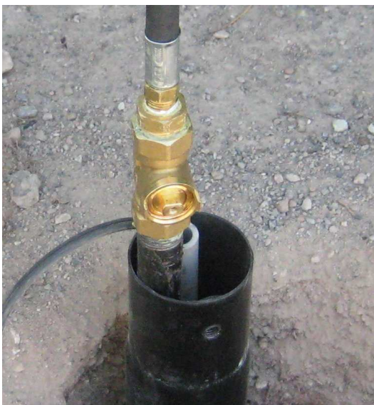
Gas ball valve with 1/2" to 1/4" reducer bushing and gas hose installed
